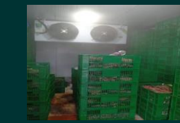
Food waste being preserved in cold room at Obunga market for processing
