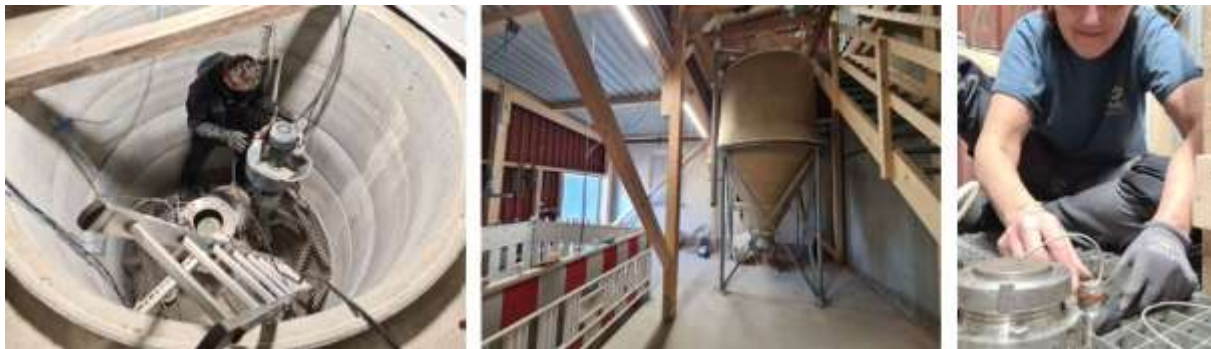
Figure 23 Underground silo during accomplishment of pressure test (left). Hermetic above ground silo (center) and installation of sensors for grain monitoring (right) (Photos: C. Müller-Blenkle, JKI)
